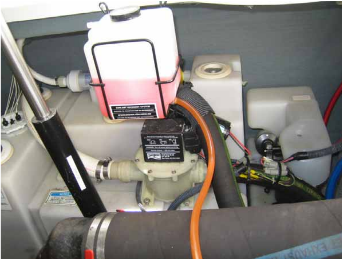
Photo 14. Vacuflush system and water tank to port in engine room.
