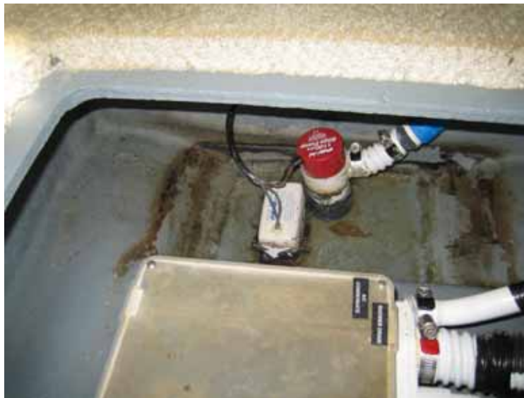
Photo 21. Bilge pump aft in engine room tested working.
